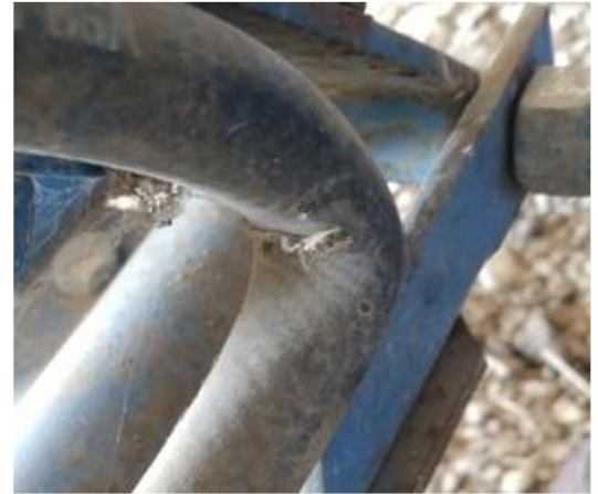
Figure 1. Crimps in hoses may lead to cracking. (Photo: Ric Bessin, UK)
